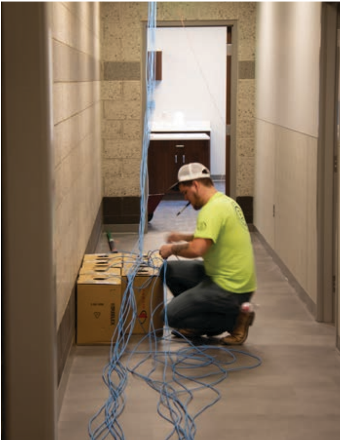
A technician runs ethernet cable for one of the Justice Center's training areas.
