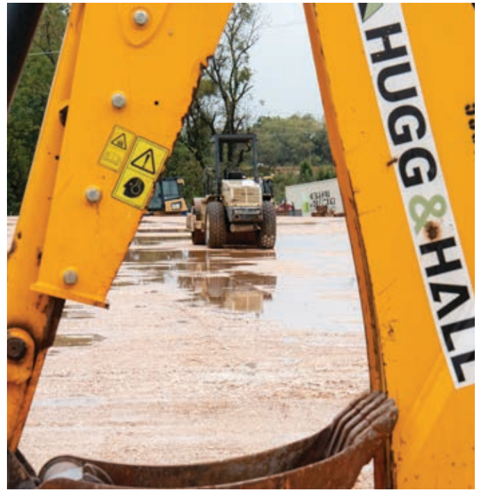
The groundwork is underway at the site of Bella Vista’s new police station and court complex, a first for the city, which incorporated in 2006.
