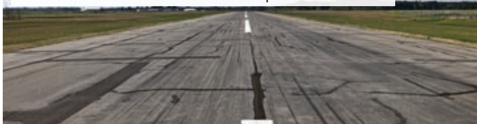
The Crossett Municipal Airport runway pre-overlay, with its cracks sealed and other repairs made.
