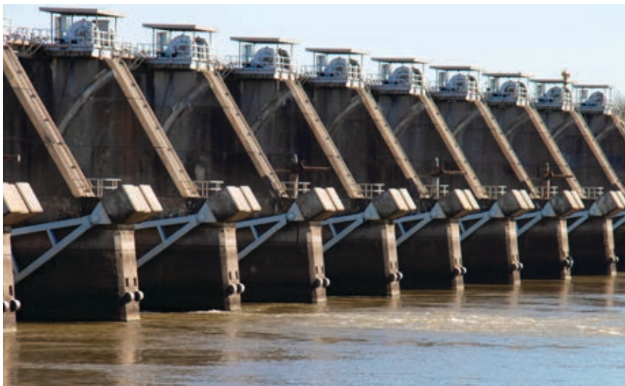
The David D. Terry Lock and Dam is part of 445-mile McClellan-Kerr Arkansas River Navigation System, which helps keep business flowing up and down the river year-round.
