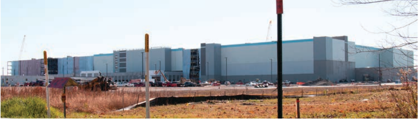
Amazon's new 826,000-square-foot facility is well underway, and CZ-USA will soon begin construction right beside it.
