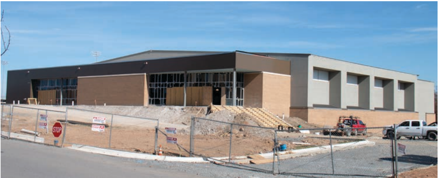
Sylvan Hills High School continues to grow, with a new arena and performance center nearing completion.
