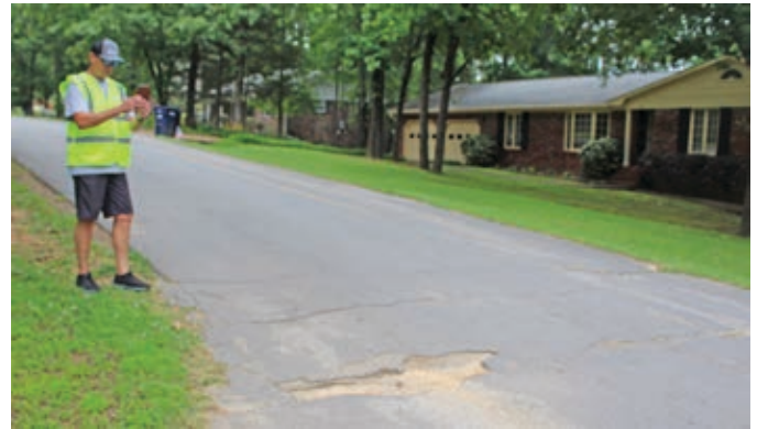
Elumbaugh takes a moment while working near the Bluff View subdivision to take a photo of an area of the street that needs maintenance work.
