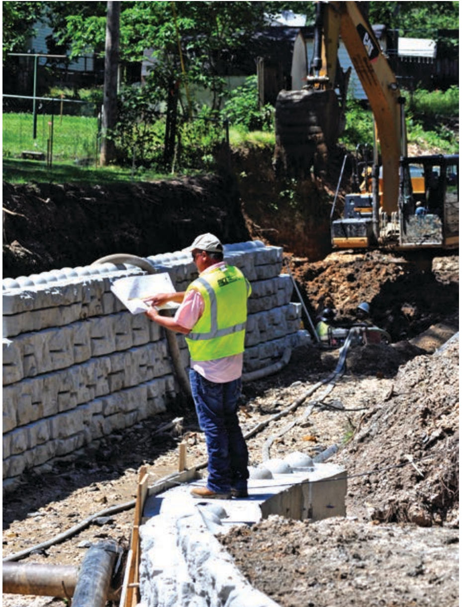
MCE's Adam Lesso observes the installation of an underground detention system in Fayetteville.
