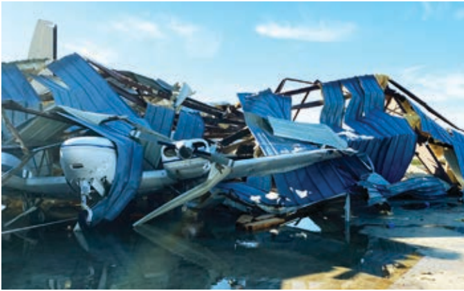
Planes and structures at the Jonesboro Municipal Airport suffered extensive damage.
