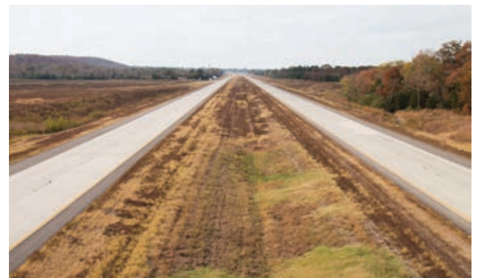
A six-mile stretch of I-49 is complete on the south side of Fort Smith near Chaffee Crossing. It will eventually cross the entire state from Northwest Arkansas to Texarkana.
