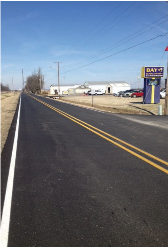
Bay students have a wonderful new school facility, but construction traffic tore up the city street. The city was able to repave with State Aid Street Program funds.
