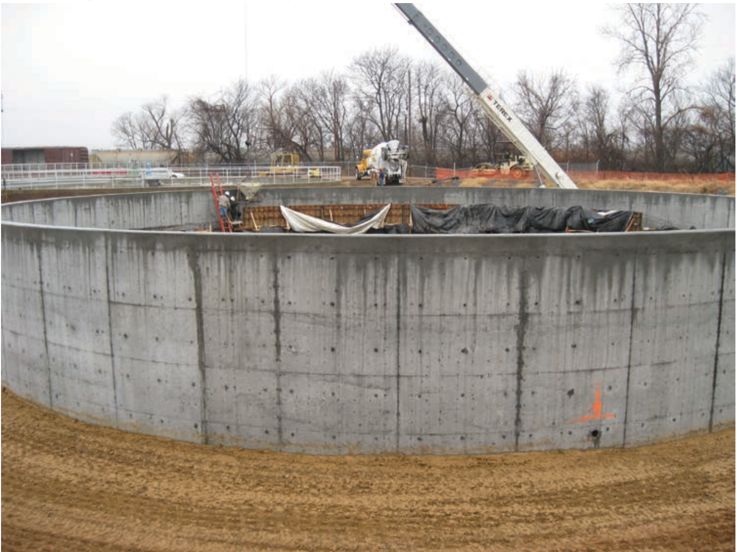
Cities can save money by taking advantage of a sales tax exemption on certain machinery and equipment used to reduce water or air pollution, as Fort Smith did with the construction of its new clarifier at the P Street wastewater treatment plan.
