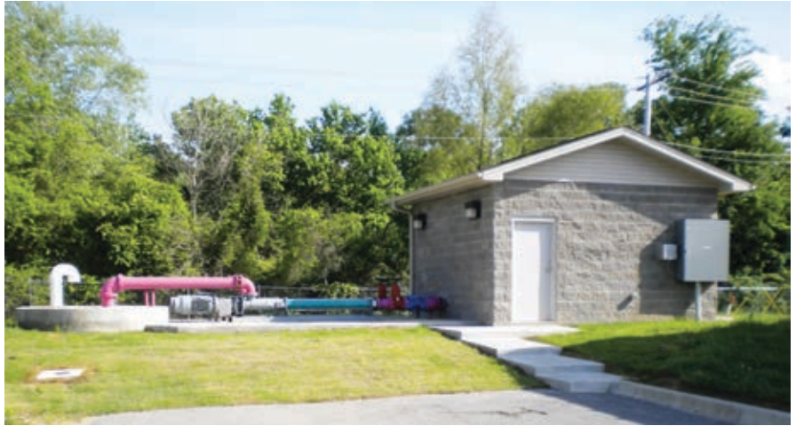
The purple pipe at Benton's wastewater utility carries non-potable water.
