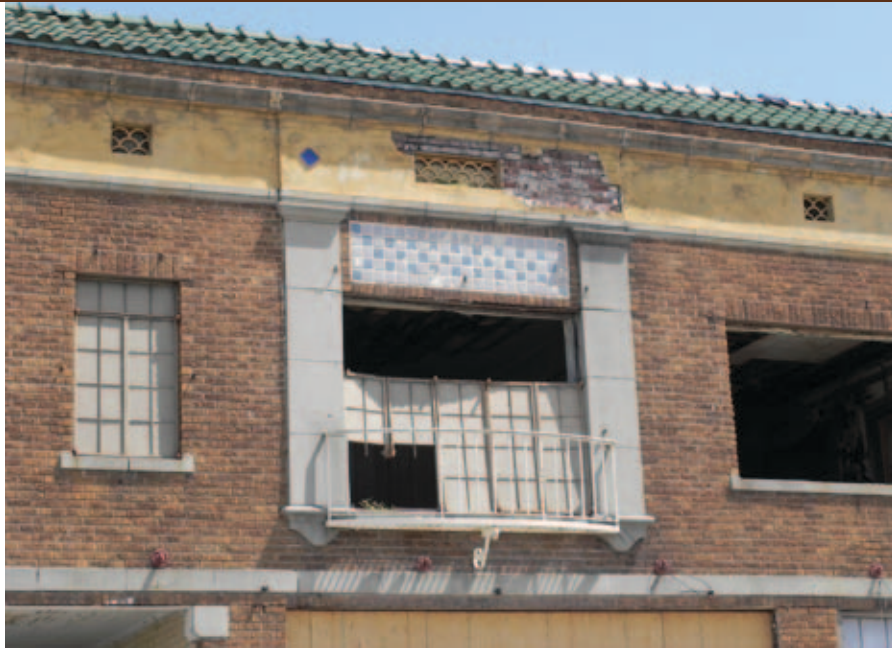
Architectural details such as this are too precious to be lost through neglect.
