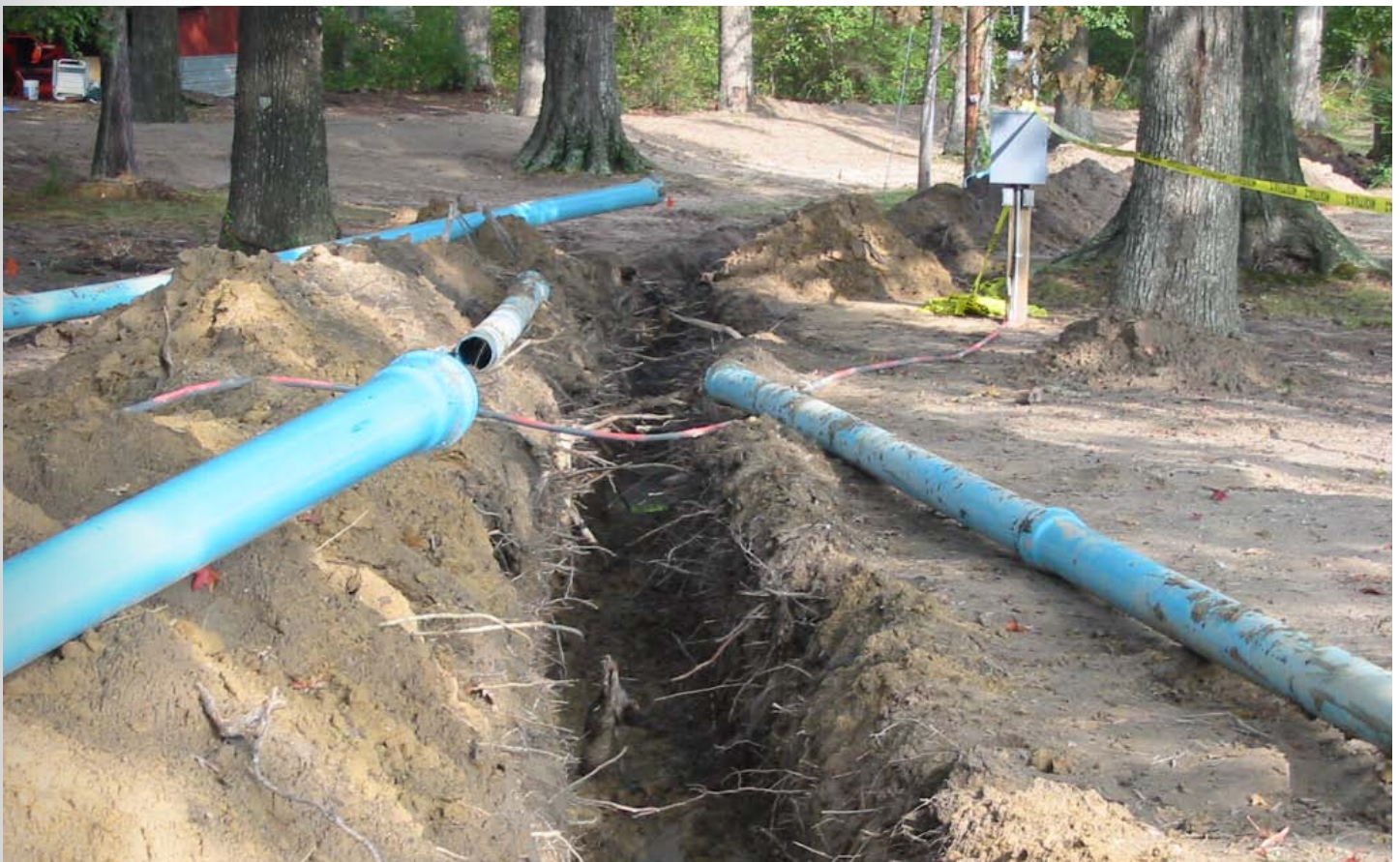
Laying utility lines is one way to compromise the strength and health of a tree's root system.
