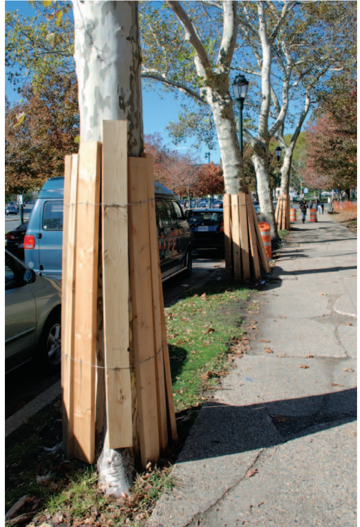
Photo 2—Q: Is this the proper way to protect trees from construction damage? A: No.
