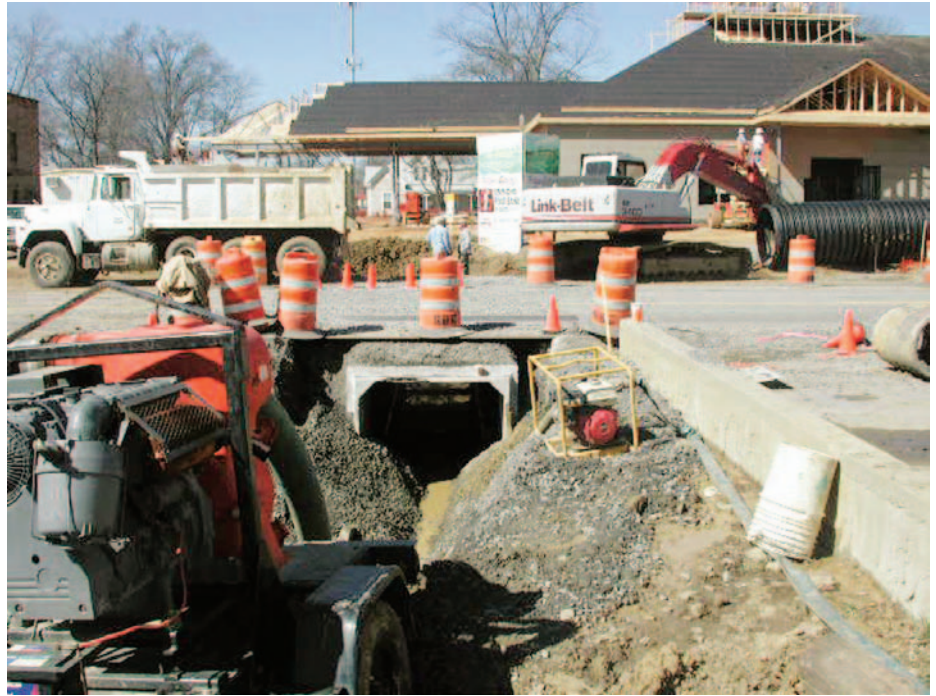
Planning and regulating can prevent costly retrofits such as this.
